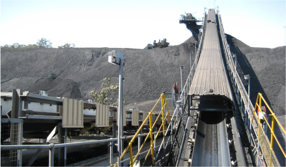
Tunnel conveyers at Glencore Bulga
